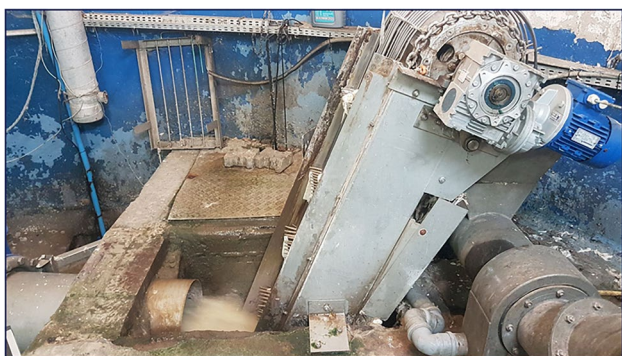
Fig. 1 An example of not hermetized process at wastewater pumping section in one of the studied WWTP
